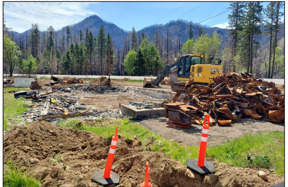
Little of the McKenzie River Clinic building in Blue River remained during cleanup operations in May of 2021.
