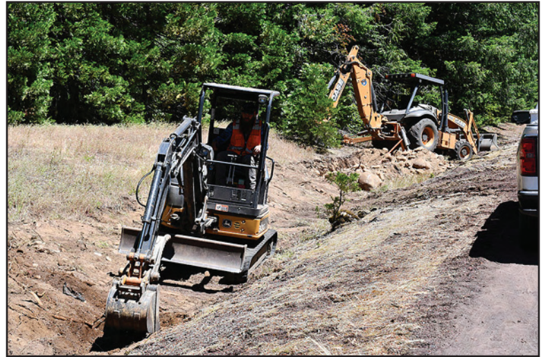
Crews from C2 Utility Contractors have been busy lately undergrounding utilities in McKenzie Bridge as part of current US Forest Service projects.
